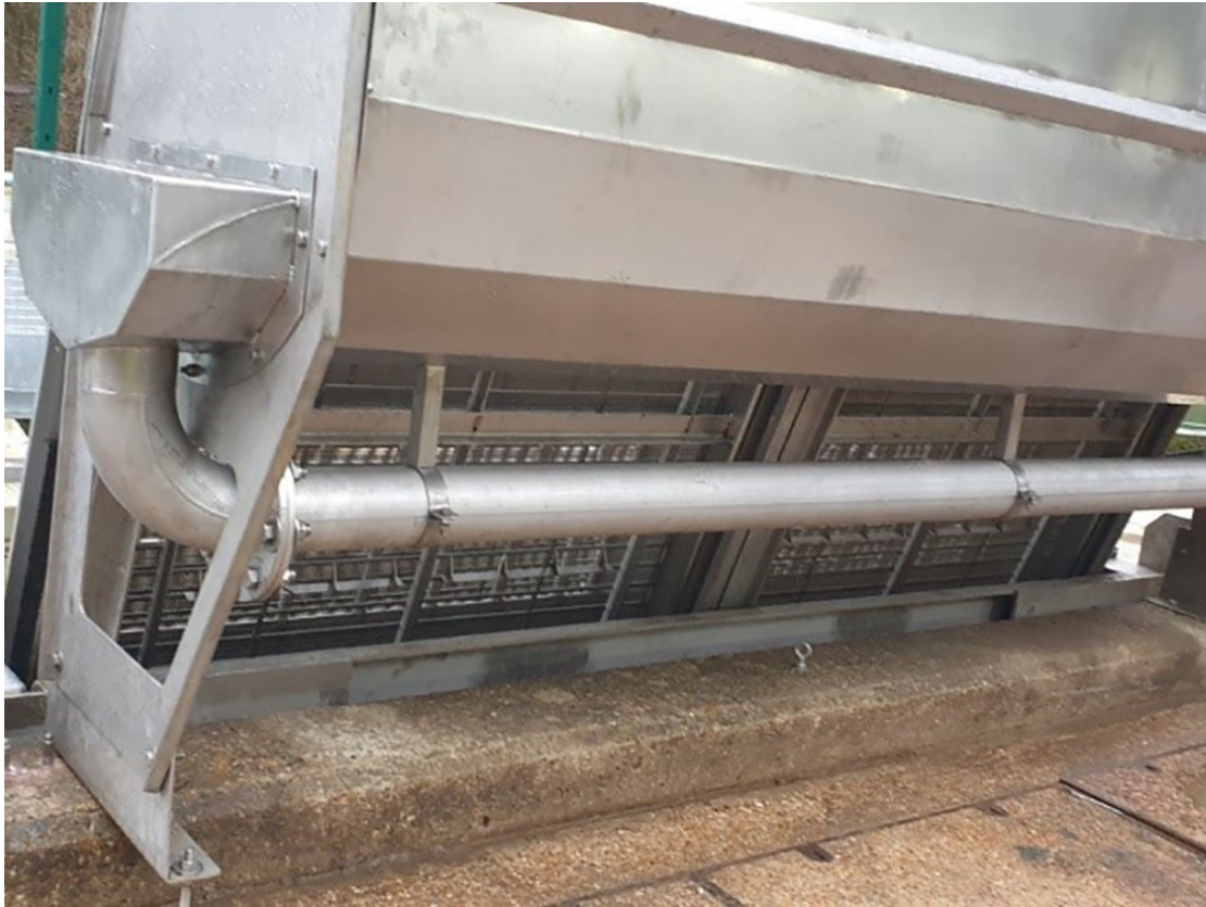
The debris flushing flow pipework underneath the Debris Trough
