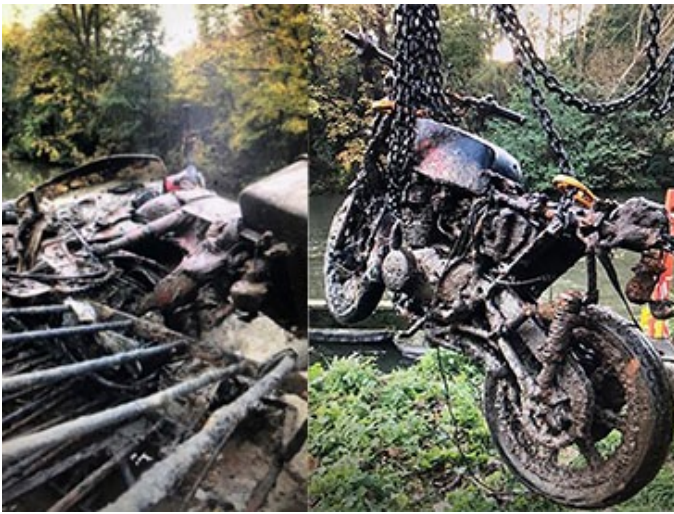
Some of the debris, including a motorbike, removed from the intake by the divers
