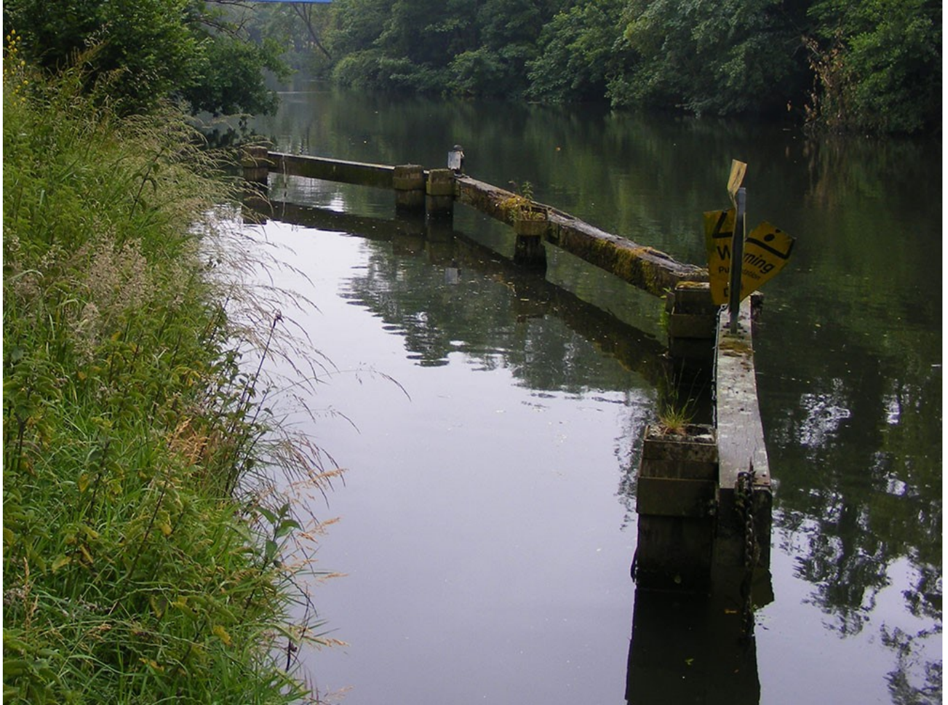
Intake location (underwater) with surrounding timber fender
